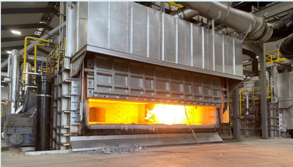
Figure 8. Thermal aluminium furnace powered with industrial fuel
